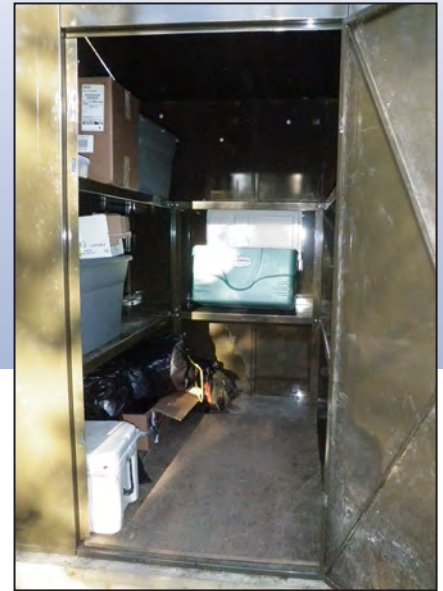
Two rows of sturdy steel shelving line the interior of each unit
